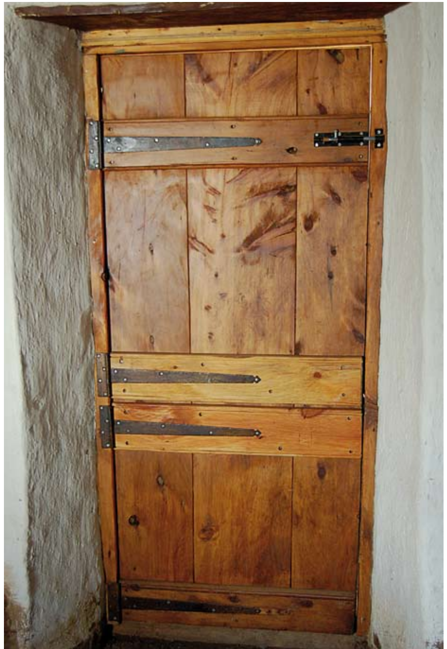
Doors and windows were replaced or refurbished, using only hand-made metal fittings
