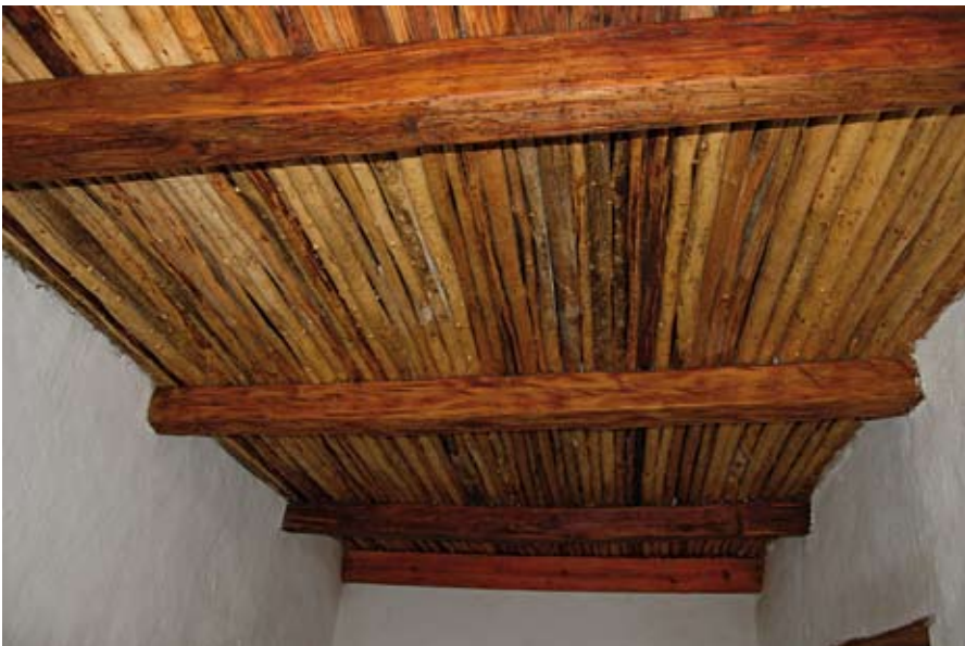
The ceiling of tree branches had a covering of lime and clay as fire protection
