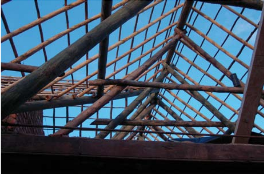
The original roof supports were tied with leather thongs and rushes, intact after 250 years
