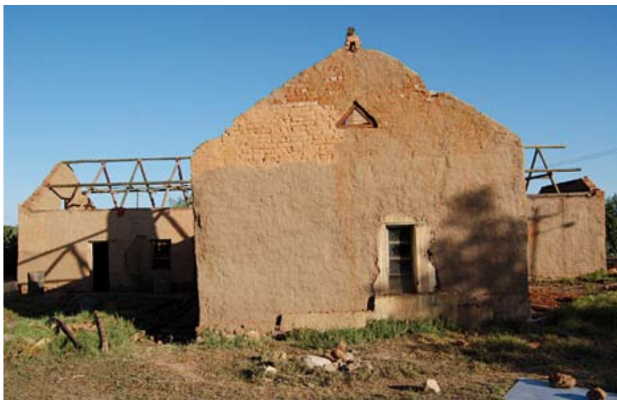
The early stage of restoration, February 2007. All the cement plaster, as well as the roof, had been removed before the process of rebuilding could begin
