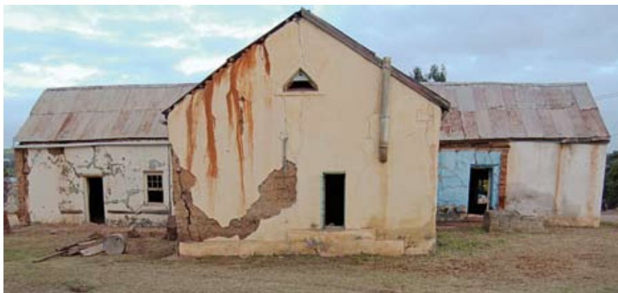
The sadly neglected building as it looked in July 2005. The leaking gutters and corrugated iron roof fed water into the top of the walls, where it was trapped by the cement plaster. The part facing the camera, the leg of the T, is the oldest part of the structure
